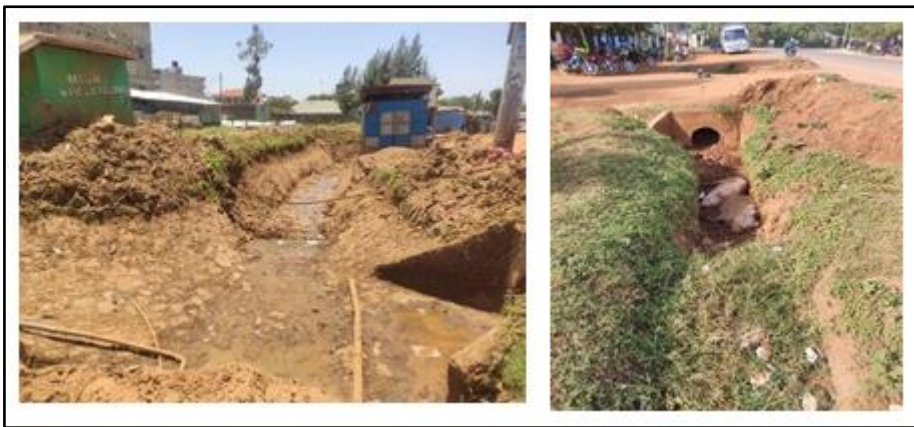
Figure 3. 5: Storm water management infrastructure
