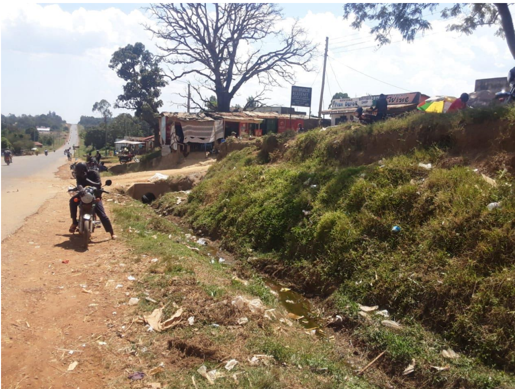
Figure 8 Storm water drain
