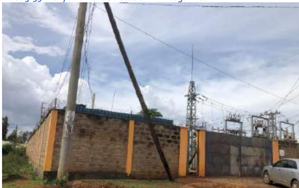
Plate 3-55: Kenya Power Sub-station in Mbaga Area
