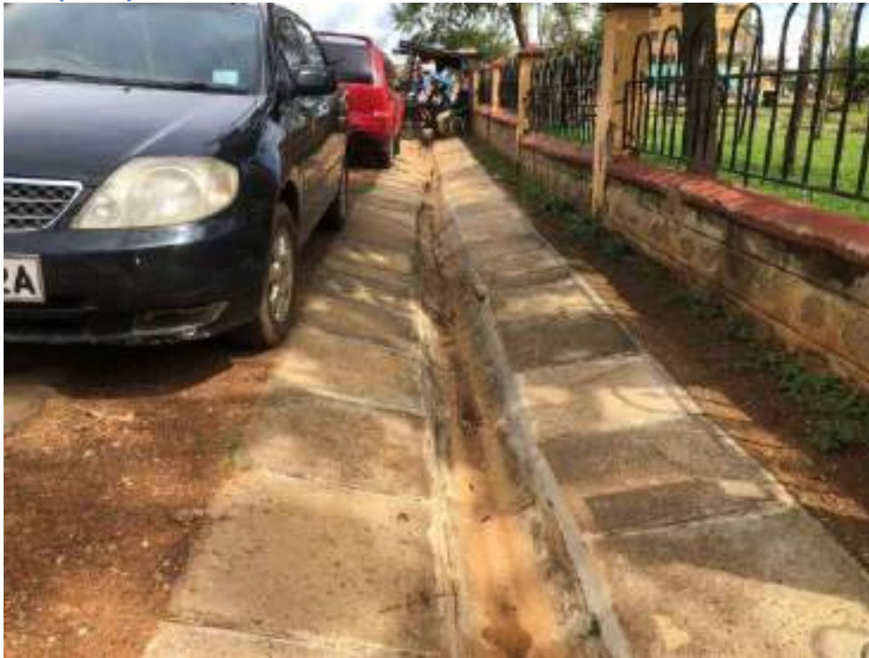
Plate 3-48: A Section of the Storm Water Drainage Along Ahindi Gardens Encroached by a Temporary Boda Boda Shade
