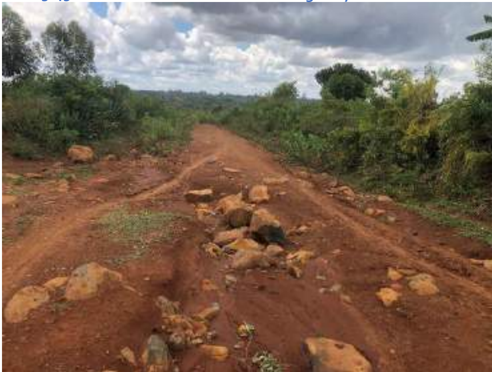
Plate 3-49: Section of An Access Road Damaged by Storm Water in Ulafu Area
