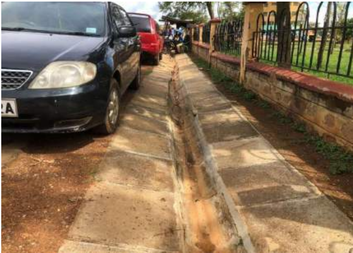
Figure 3-2: Storm Water Management Infrastructure
